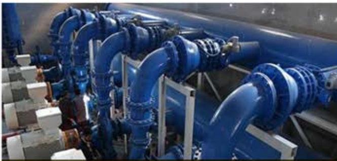
Water transmission line, pumping station, reservoir, and access road to the water transfer project from Dosti Dam to Torogh Dam
