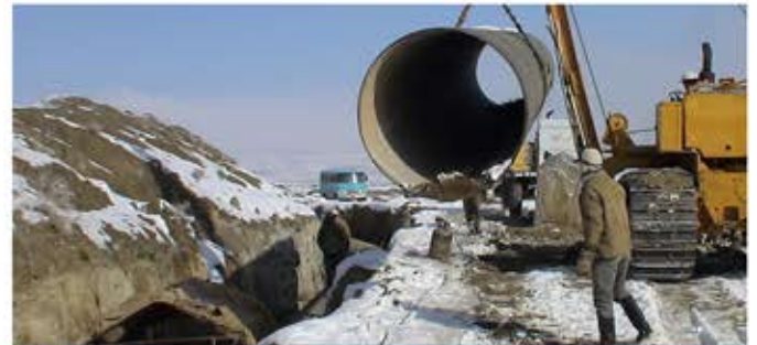
➤ Water transmission line and reservoirs 3, 4, 5 and cathodic protection of water supply from Kamal Saleh dam to Arak
