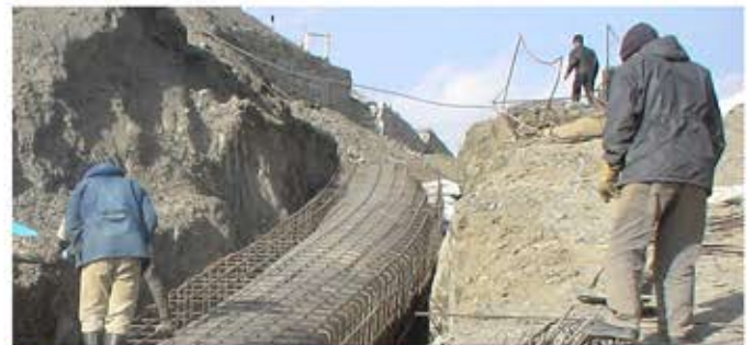
Execution of transmission line, access road and cathodic protection of Semnan water supply project from Roozieh fountain
