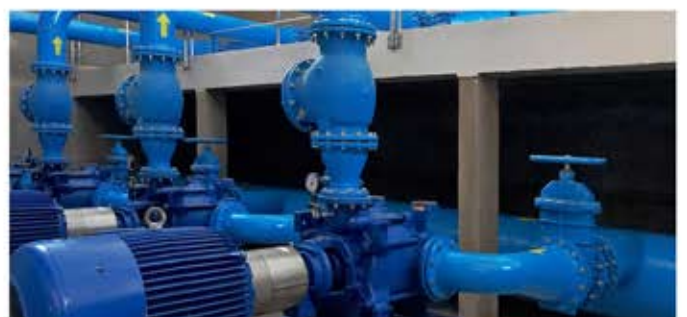
The main pumping building of Jofa plain, electrical and mechanical equipment
