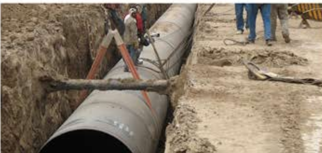
Water transfer line from Abadgaran three ways to C-zone reservoir - Mashhad - 5th section
