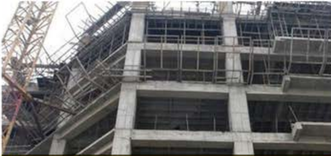
Execution of operations in the administrative building of the General Inspection Office of Hamadan Province
