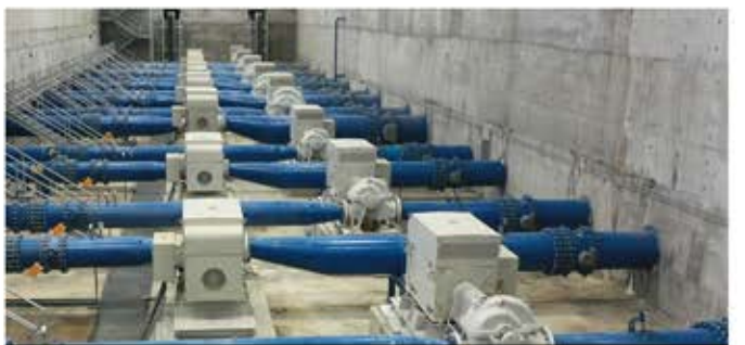
Procurement, Displacement, Installation, and commissioning of tank equipment for a new pumping station and treatment plant in Nahand
