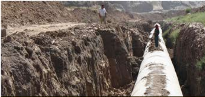
Completion of the first section of the transmission line and landscaping of the 180,000 reservoirs and the electrical installation of the Taleghan to Karaj water transfer project
