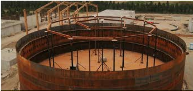
➤ Design, Purchase, Construction, Installation, and Commissioning of water treatment plant received from the south of Tehran and its transfer in the refinery area
