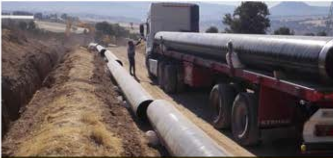
Transferring water from Ilam Martyrs Dam (Galal) to Petrochemical Company
