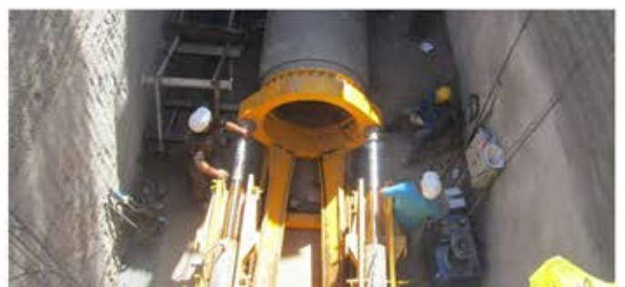
Construction of wastewater treatment plant and sewage transmission line with a diameter of 1200 mm and a length of 10 km in Birjand
